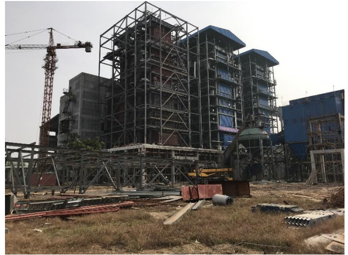
*One operating boiler and one spared Source: PSR
