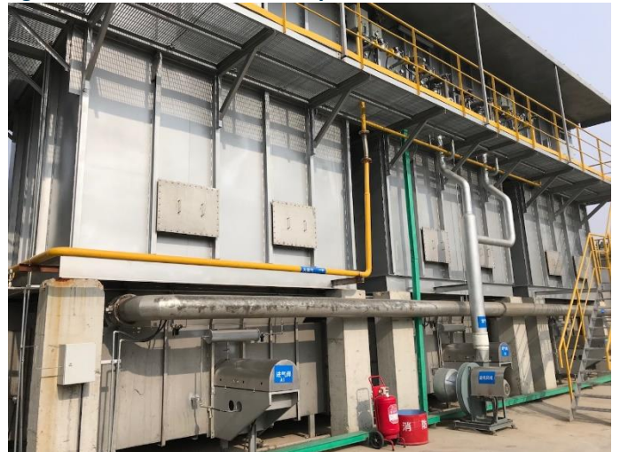
Figure 28: Odor collection facility
