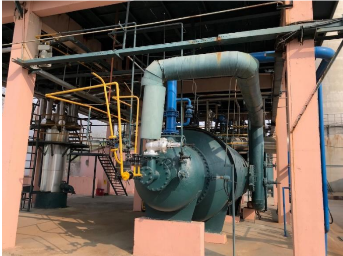
Figure 25: Hydrogen sulphide recycling facility
