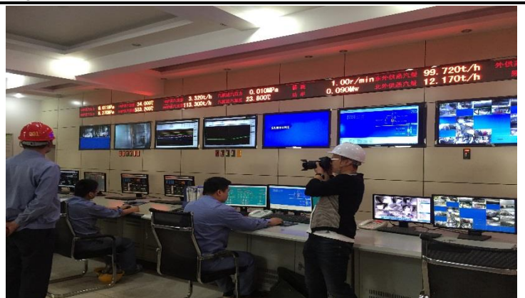
Fig 19: Centralised control room
