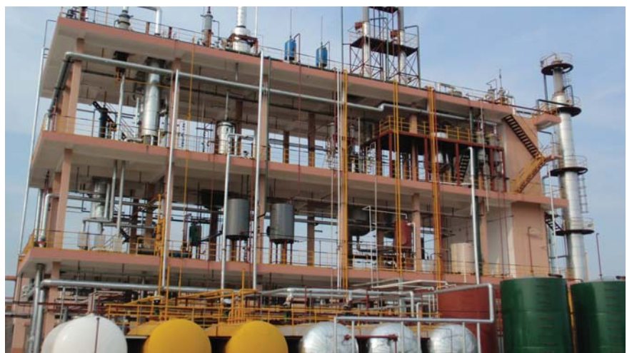
Anti-oxidant TMQ Plant
