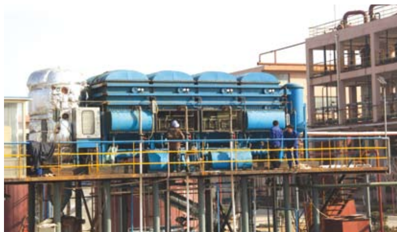
Waste water treatment plant – Distillation Machine
