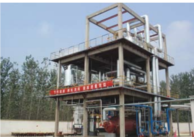
Sulphur Gas Recycle Facility
