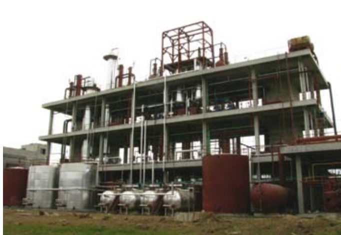
15,000-ton 6PPD Plant at Shanxian Facility 2
