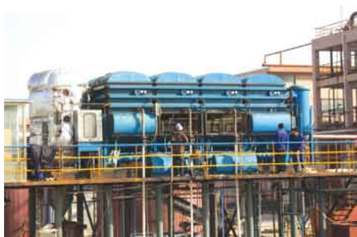
Waste water treatment plant - Distillation Machine at Shanxian
