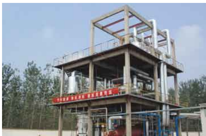
Sulphur Gas Recycle Facility at Shanxian
