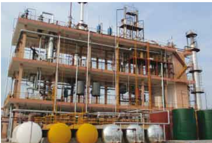
10,000-ton Anti-oxidant TMQ Workshop plant at Shanxian
