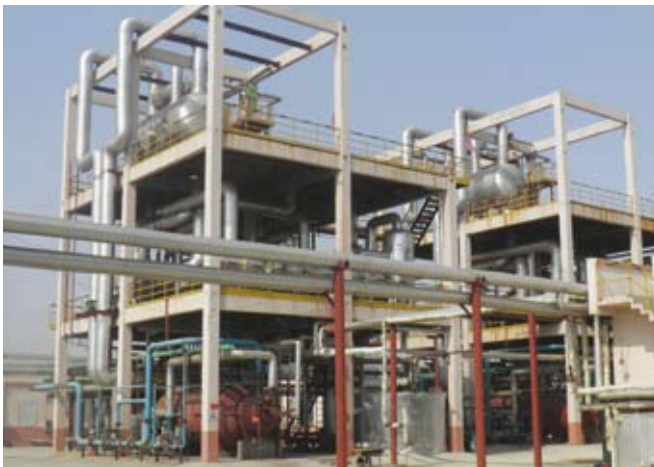
Sulphur Gas Recycle Facility at Weifang
