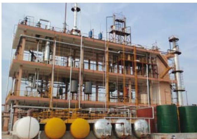
10,000-ton Anti-oxidant TMQ Workshop at Shanxian
