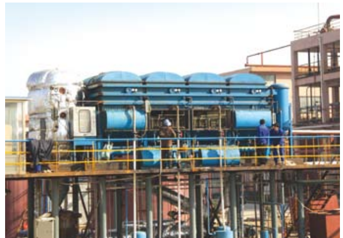
Waste water treatment plant – Distillation Machine at Shanxian
