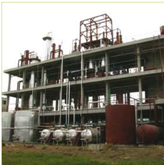
15,000-ton 6PPD Plant at Shanxian Facility
